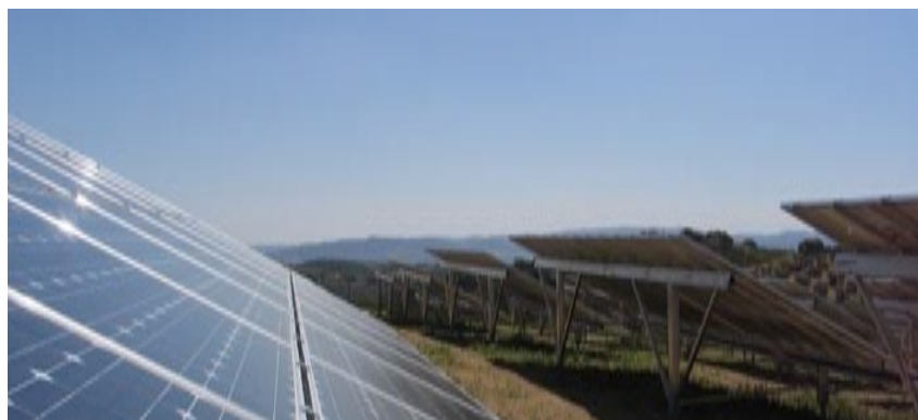
Photovoltaik-Projekt in Loja, Andalusien
