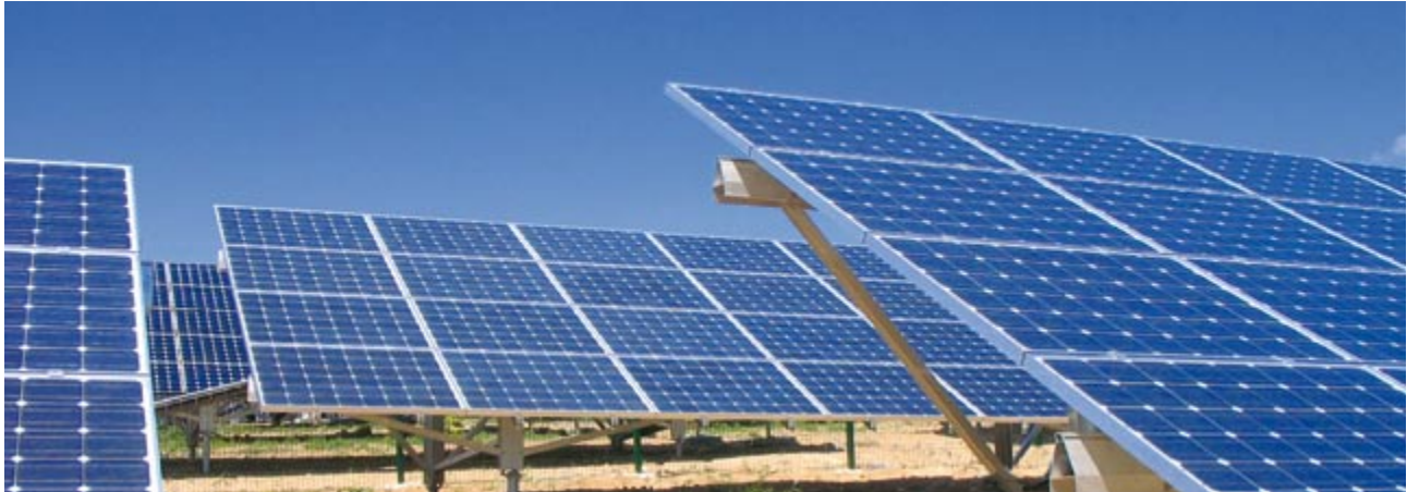
Solar park in Loja, Andalusia
