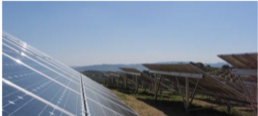
Photovoltaic project in Loja, Andalusia
